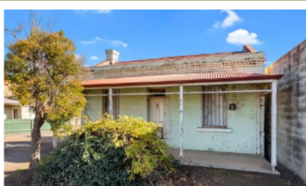
92 Victoria Street Eaglehawk has been left vacant for many years and is one of the many homes that has been left to the elements for survival. Photo: Bendigo Branch
