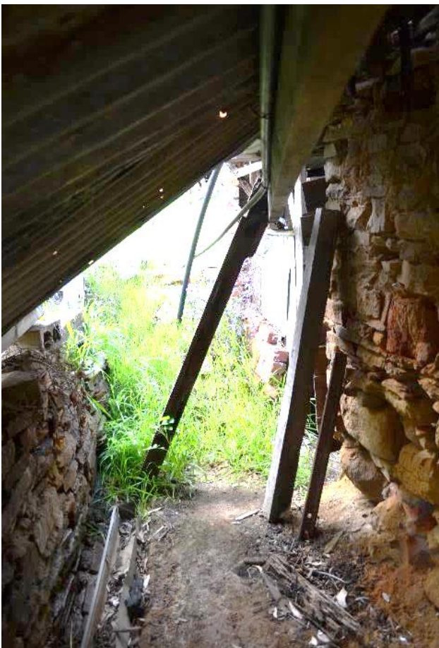
Figure 7: By 2017 the verandah had collapsed and the condition of the wall had worsened and was in danger of collapse. Photo: supplied
