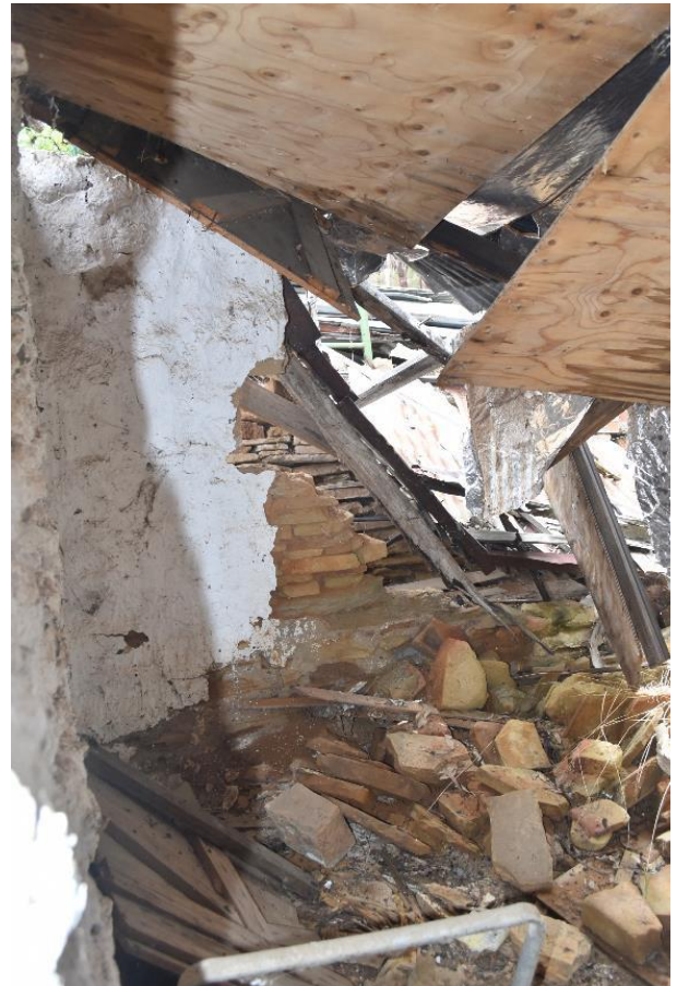
Figure 8: By 2022 the wall and roof had collapsed. Viewed from the inside. The outside is now inaccessible due to the collapsed roof and wall. Photo: supplied
