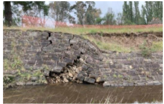
Flood damaged section of the Chewton Wall in the Castlemaine Diggings Heritage Park. Source: Chewton Chat February 2025
