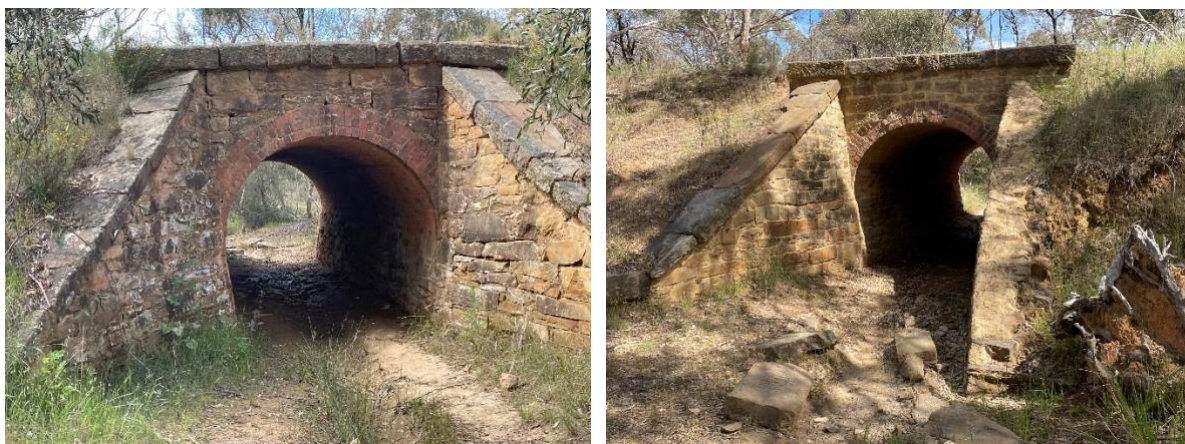
Two views of this Spring Gully stone bridge showing the large supporting buttresses and interesting tunnel shape. Image supplied
