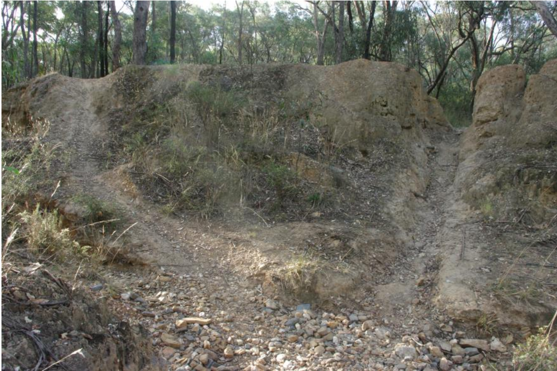
PHOTO 1. ILLEGAL MOUNTAIN BIKE TRACKS OVER AND THROUGH A HISTORIC GOLDFIELDS MINING DAM WALL. BENDIGO REGIONAL PARK.
