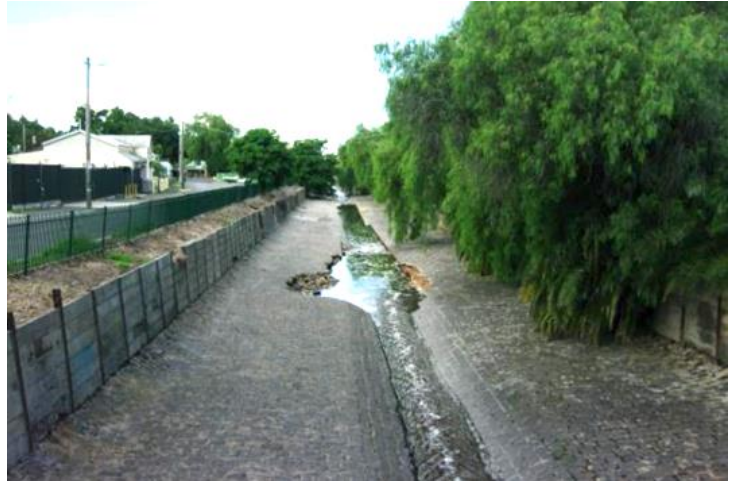
Bendigo creek bed bluestone blocks broken away and washed downstream. 9 Jan 2024. Image: Norm Stimson
