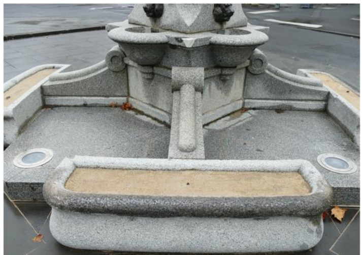
Cleaning has occurred but the historic photos and story has not been reinstalled. Image: Branch 2022
