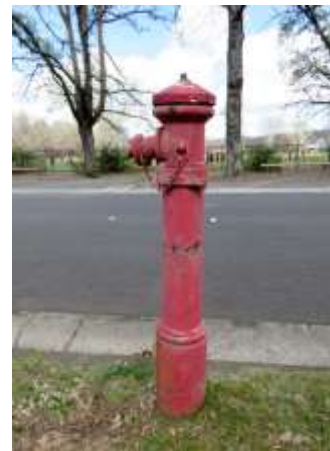
Complete Pillar Hydrant, opposite 46 New South Wales Crescent, Barton
