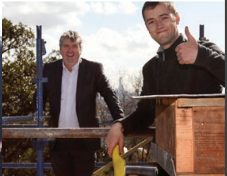
Martin Purslow supporting the use of best practice heritage trade skills on the roof at Rippon Lea.
