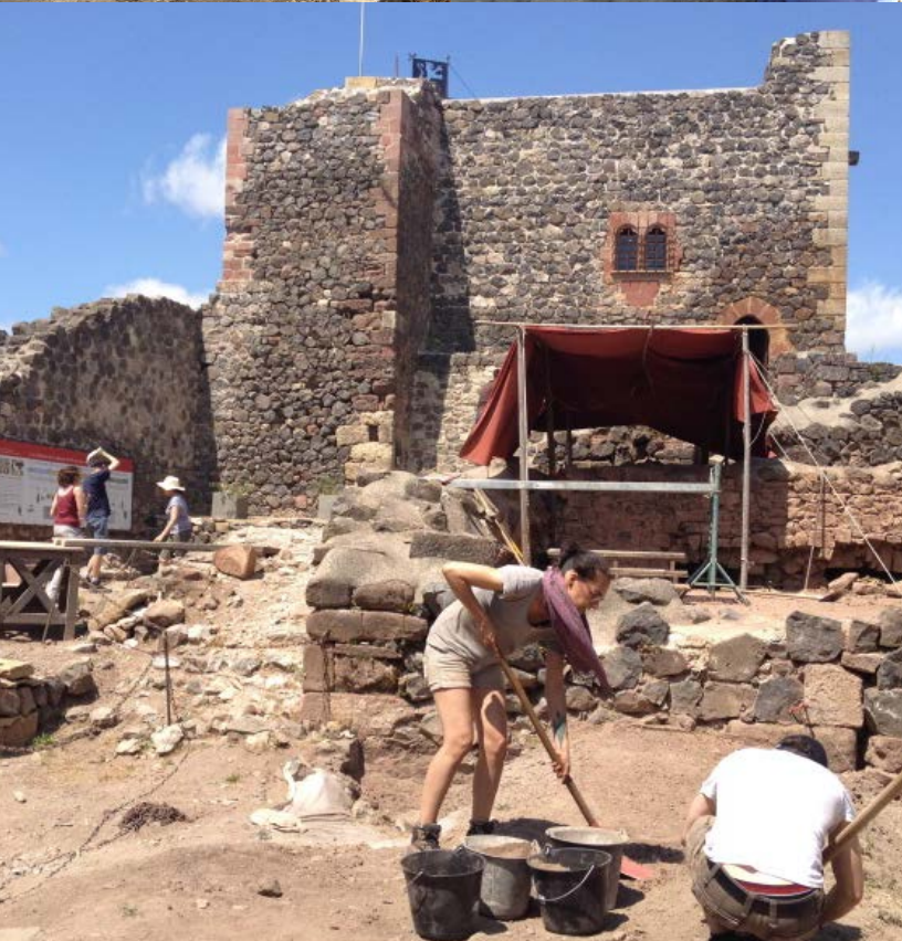
Rebuilding of a wall at Montalet Castle and excavations at Calmont d'Olt Castle
