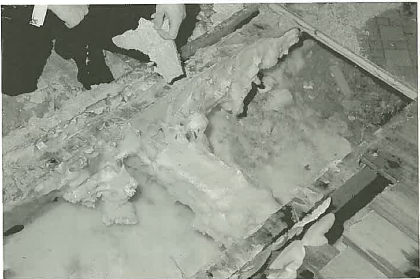
Dense mycelium mat of Serpula lacrymans beneath a poorly ventilated and badly decayed floor.
