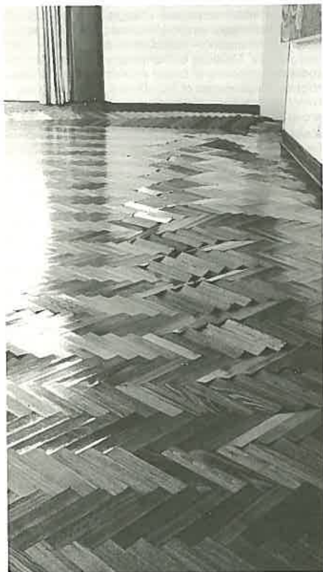
Parquetry floor which has been allowed to become damp, has swelled and lifted.
