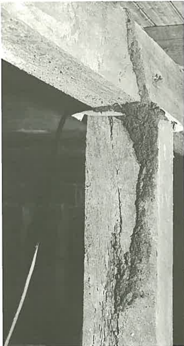
Subterranean termite (White Ants) reach susceptible timber in a building by constructing mud-covered shelter tubes to connect their nest with their source of food.
