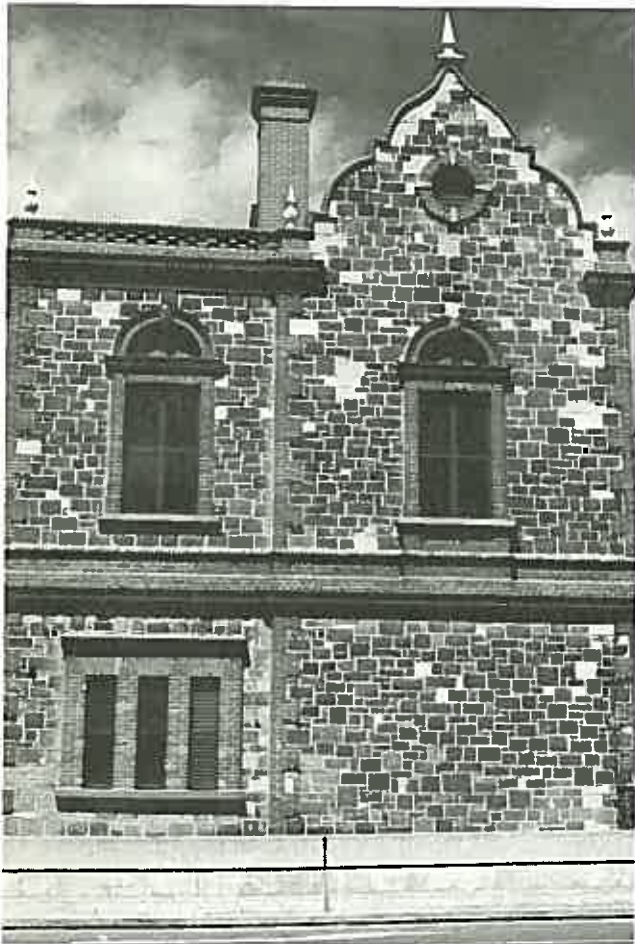
Plate 7: An unattractive contrast may be produced between clean replacement stone and old soiled stone. The original Tea Tree Gully sandstone of the Old Legislative Council Building, Adelaide, is still grimy after washing in 1980. The light blocks are of clean Sydney sandstone.
