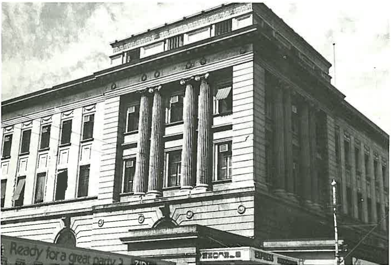
Plate 4: Aspect and exposure control the distribution of soiling. The exposed, west-facing wall of the stucco Adelaide Railway Station (on the left) is light coloured and comparatively clean as the surface is crumbling and self-cleaning. The southern wall (in shadow) is much sounder and more grimy as the dirty original surface still remains.
