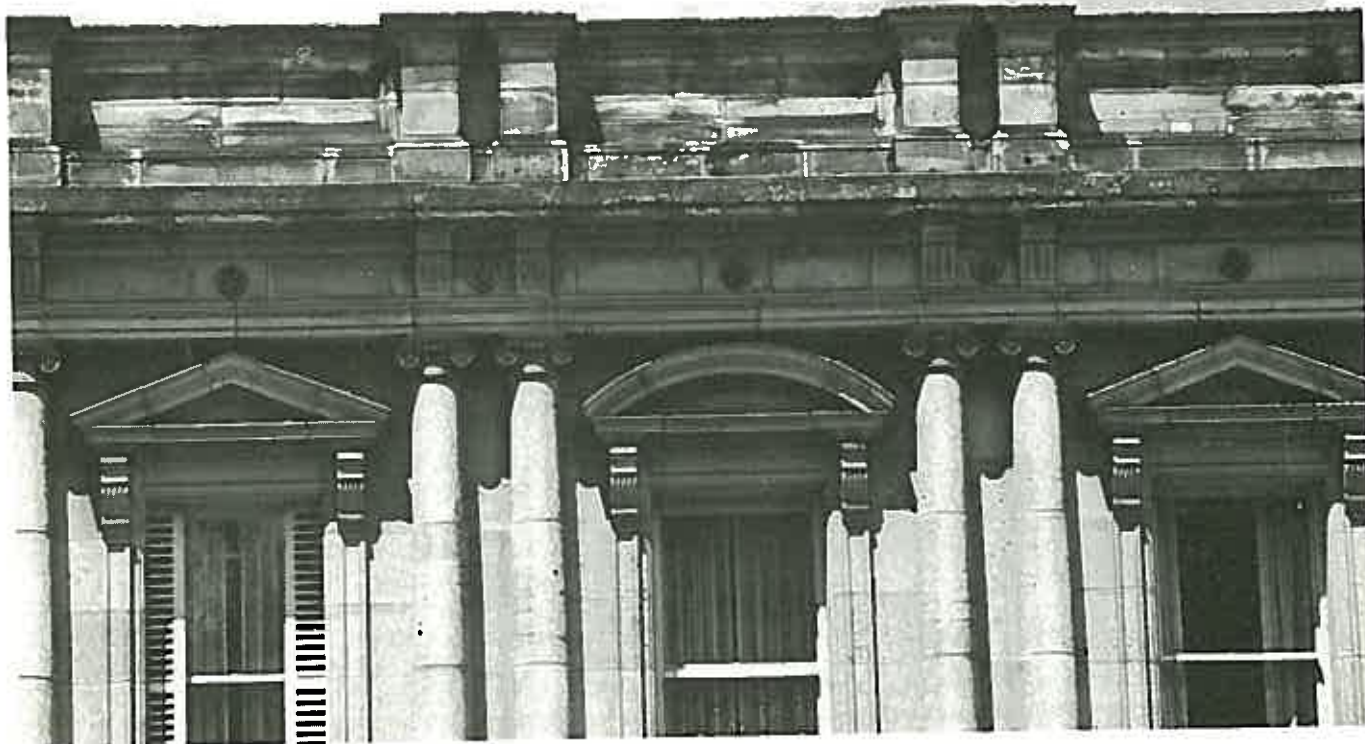
Plate 2: Architectural detailing controls the distribution of soiling. The sandstone parapet is typically stained and the soffit of the cornice with its open joints is decayed and encrusted with a black gypsum-bearing deposit.
