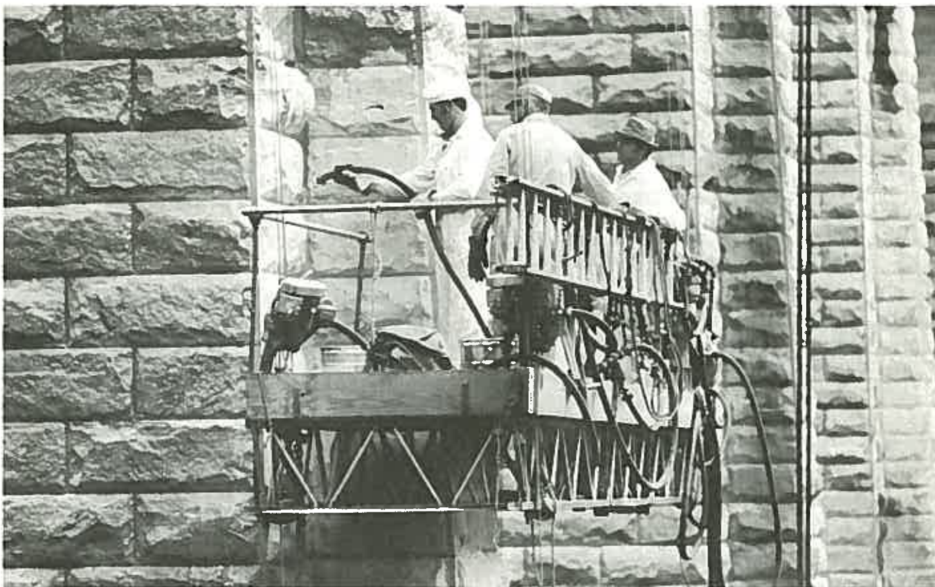
Plate 13: Dry sandblasting of the Sydney sandstone in the piers of Knapsack Gully Bridge, New South Wales. The method is effective but damages the surface. Protection from airborne silica dust for the operators is inadequate.
