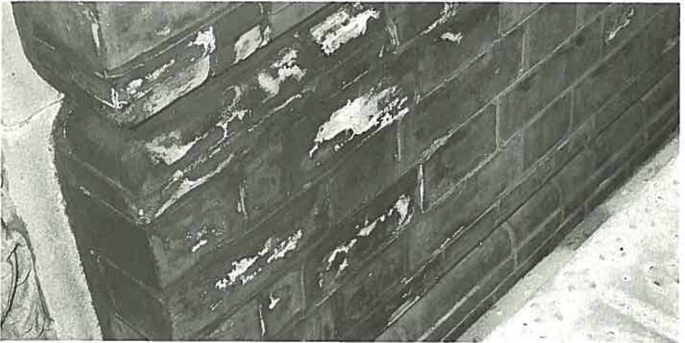
Plate 8: Chemical cleaning can be effective and non-damaging, but the use of caustic alkali on these bricks in the Bank of New South Wales, Sydney, has left salt staining and efflorescences even after repeated washing.
