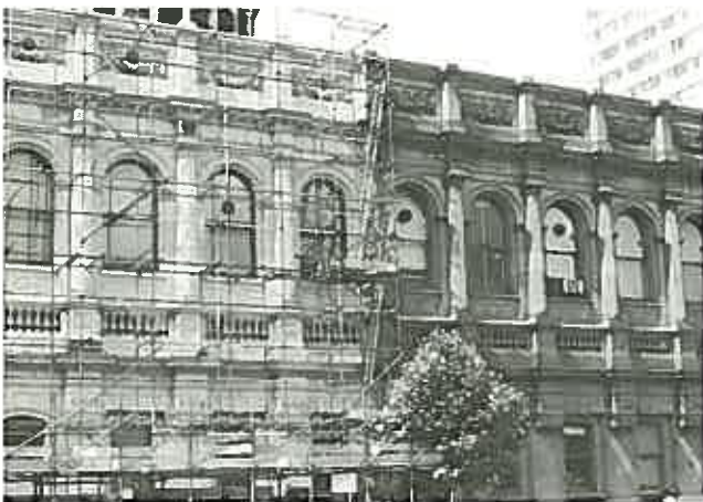
Plate 3: Cleaning may produce a marked improvement in the appearance of a building as the contrast between the cleaned and uncleaned sandstone of the Melbourne Supreme Court shows. However, harsh cleaning may have only a temporary effect in polluted urban atmospheres.
