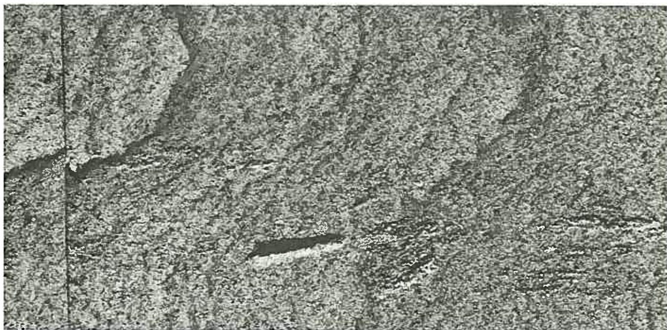
Plate 10: Manual abrasion (carborundum block) of sandstone can leave the surface scratched and pitted. The surface of this Helidon sandstone on the Anzac Memorial, Brisbane, has been badly damaged.
