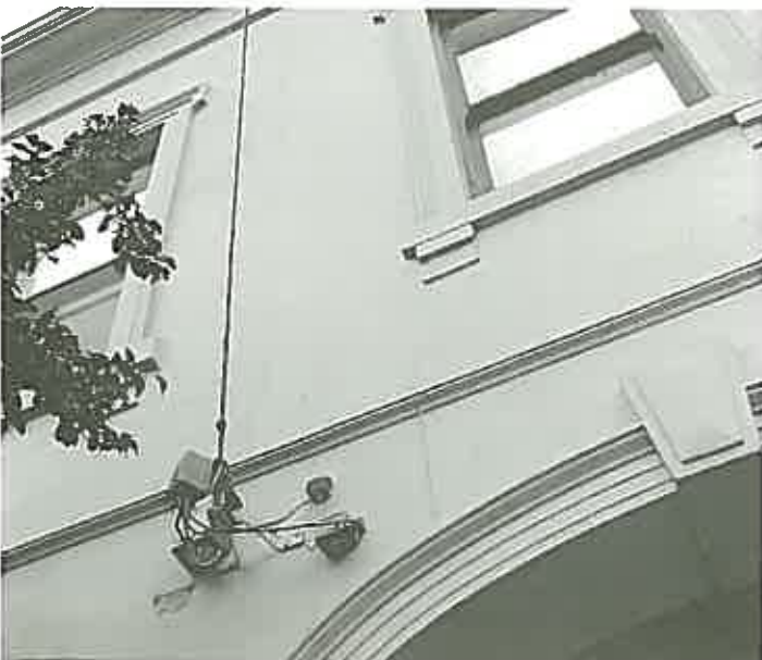
B. Facade of Falconer Terrace, crack 1 is to the left of the party wall line and crack 2, as shown in the detail, is to the right of its party wall. This shows that part B is earlier than parts A and C. This is confirmed by documentary evidence which indicates that A [no 50] dates from 1870, B [nos 48, 46, 42] from 1866, and C [no 42] is from 1872. Numbers 38 and 36, off the picture to the right, date from 1880 and 1884 respectively.
