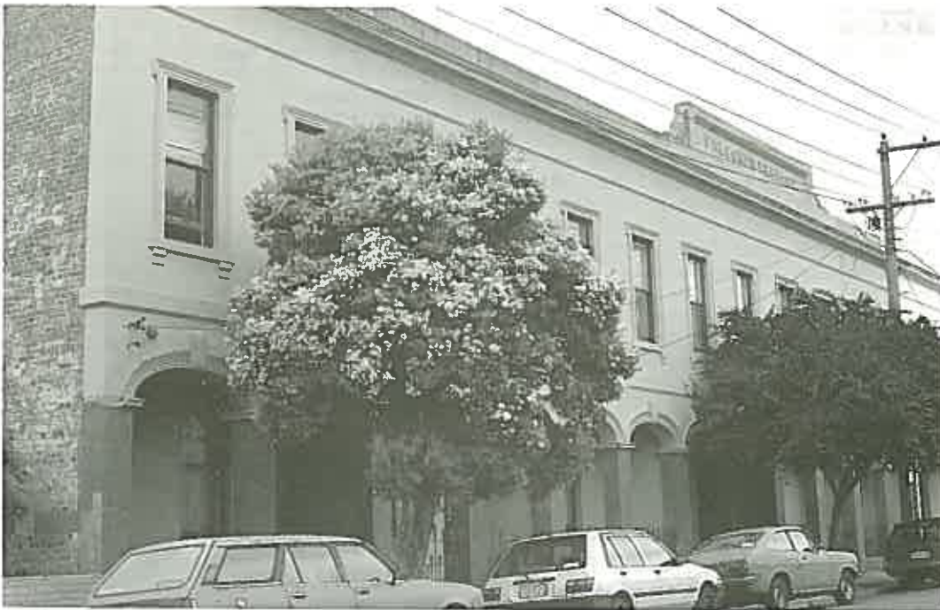
A. Detail of Falconer Terrace, 36-52 Napier Street, Fitzroy: the location of cracks in this apparently uniform facade indicates the different dates of construction. The crack or discontinuity at the junction of numbers 42 and 44 is to the right of the party wall, indicating that number 44, to the left, is the earlier portion.
