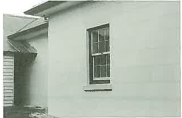
The walls of this building are brick plastered and lined out to simulate ashlar. Only the window sill is sandstone. (Cooma Cottage, Yass, N.S.W. Restoration architect: Clive Lucas)
