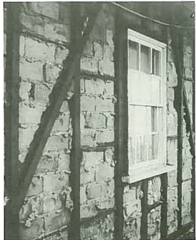
This early cottage in Sydney has had its external weatherboards removed revealing its brick nogged construction. The boards should be restored. ( Cottage, 45 Glebe Street, Glebe, Sydney. )
