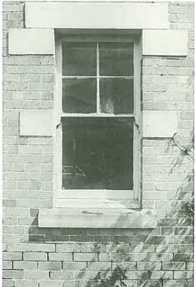
A typical example of the effect of rising damp on the exterior of a brick building. ( Beulah Vista, Church Street, Canterbury, Sydney. )
