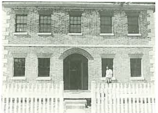
After hacking of the cement render and rebuilding the face of the wall and restoring the stone dressings and tuckpointed the brick arches the house is recognisable again as Georgian. ( Restoration architect: Clive Lucas. )
