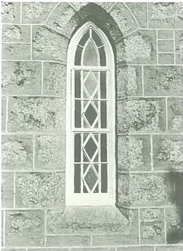
In this example tuckpointing has been used to make the masonry appear finer than it is. ( Uniting Church, Beechworth, Victoria. )
