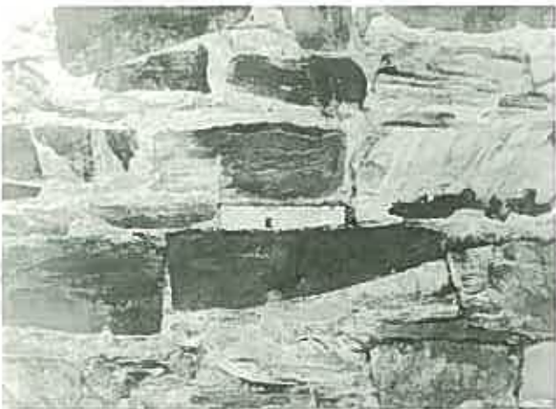
A rubble garden wall before restoration. (Brewery, Burra, South Australia.)
