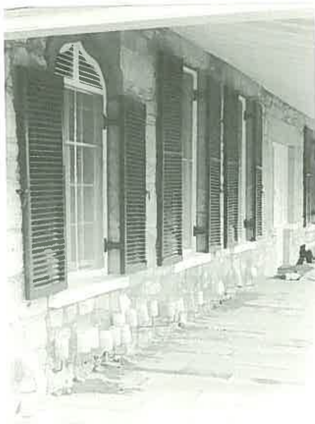
Injecting walls with a fluid is one patented attempt at stopping rising damp. (Malahide, Fingal, Tasmania.)
