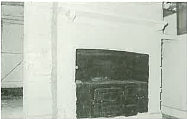
Face brick interiors were almost always painted. ( Kitchen in terrace house, 26 Derwent Street, Glebe, Sydney. )
