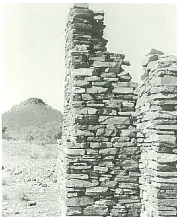
Walls built of random rubble collected from the countryside in its most basic form. (Miner's cottage, Arltunga, Northern Territory.)
