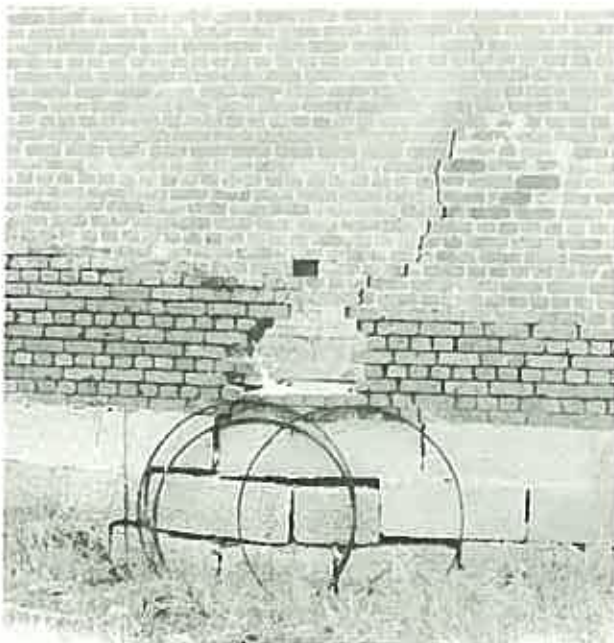
Inadequate footings plus the effects of rising damp lead to wall collapse. (Coolangatta, Berry, N.S.W.)
