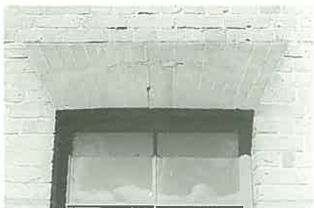
Early brick arches were often covered in red ochre and tuckpointed. As with all tuckpointing it is an attempt to make the jointing appear finer than it is. ( Outbuilding, Strathmore, Nile, Tasmania. )
