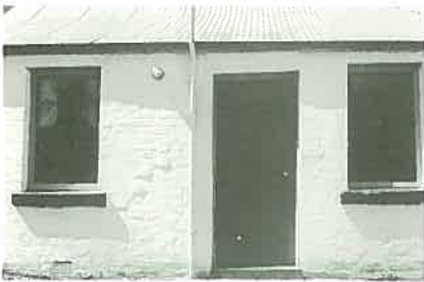
A fresh coat of limewash is the best traditional finish for soft sandstock brickwork. (267 George Street, Windsor, N.S.W. Restoration architect: Clive Lucas.)
