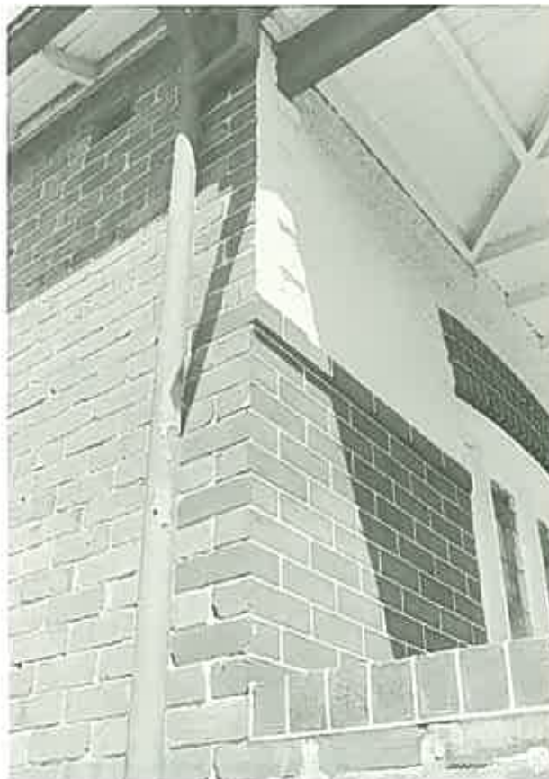
The emphasis on the front wall continued into the period between the wars, better quality bricks and tuckpointing being popular. ( Cottage, Haberfield, Sydney. )
