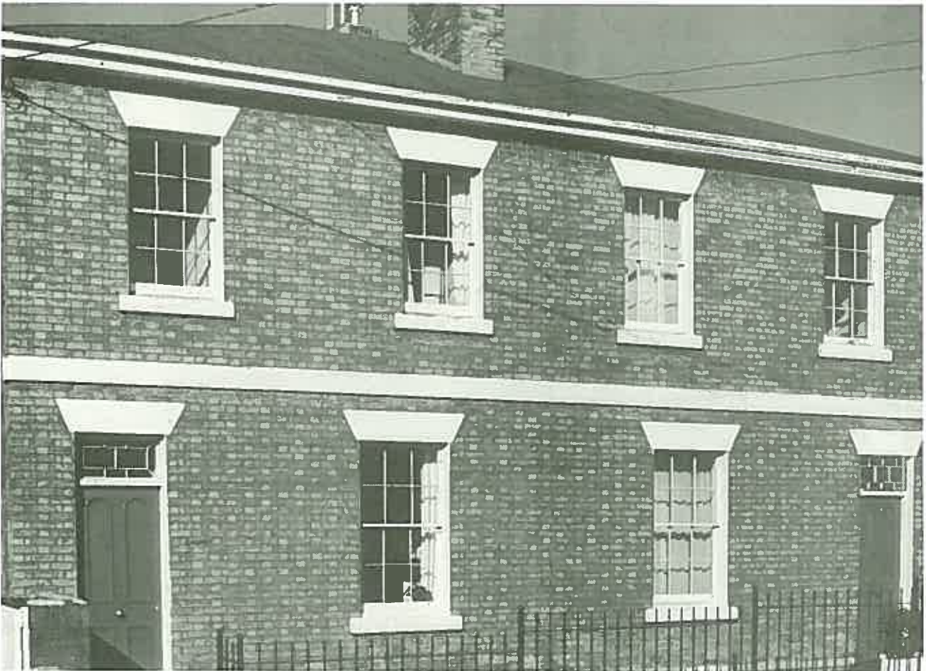
Finished in red ochre and oil to help waterproof the porous brickwork. (50 Hampden Road, Battery Point, Hobart. Photo: Wesley Stacey.)
