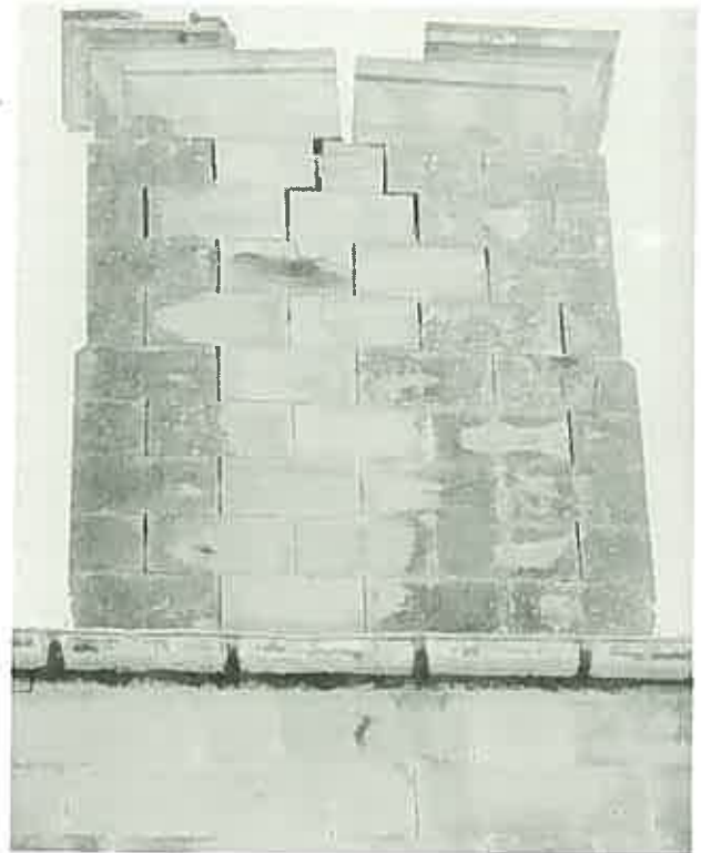
The coping has long gone and the chimney has reached the point where collapse is imminent. (Aberglasslyn House, Maitland, N.S.W.)
