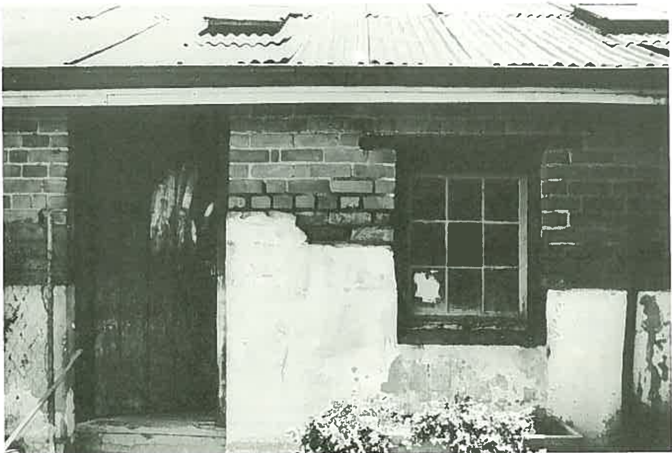
Rendering walls only drives the rising damp further up the wall. (Faversham, York, W.A.)
