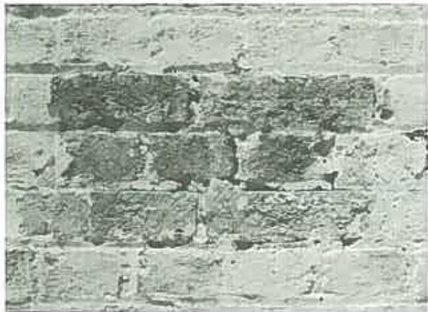
Removing paint off sandstock brickwork by water pressure removes the paint but also the soft jointing and makes the wall very wet. It would have to be repointed.
