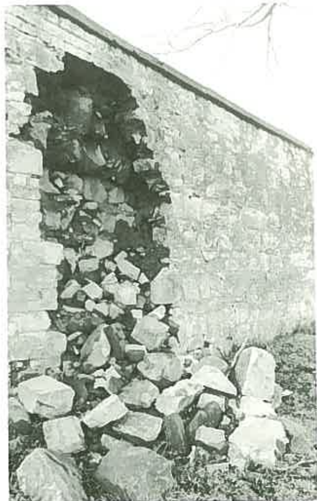
The breakdown of the coping has led to water entering the core which ends with collapse. ( Garden Wall, Rosedale, Campbell Town, Tasmania. )
