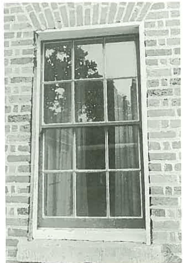
An example of badly repointed brickwork. Cement has been used and there has been no attempt to strike the joints. ( Bob's Hall, Lancer Barracks, Parramatta. )
