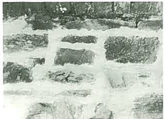
The technique used for repointing the wall shows no respect for the original material or technique. The result of unthinking repair is a disaster. (Brewery, Burra, South Australia.)
