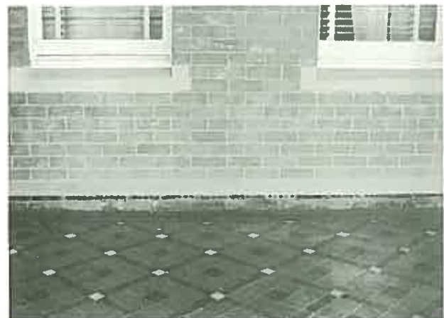
A similar dampcourse to Taylor's employed in a New South Wales Public building. (Kenmore Hospital, Goulburn, N.S.W.)
