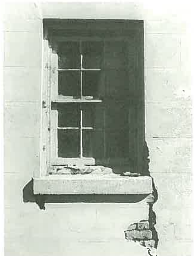
A brick wall rendered in imitation of ashlar. Only the window sill is sandstone. (Richmond Villa, Campbelltown, N.S.W.)
