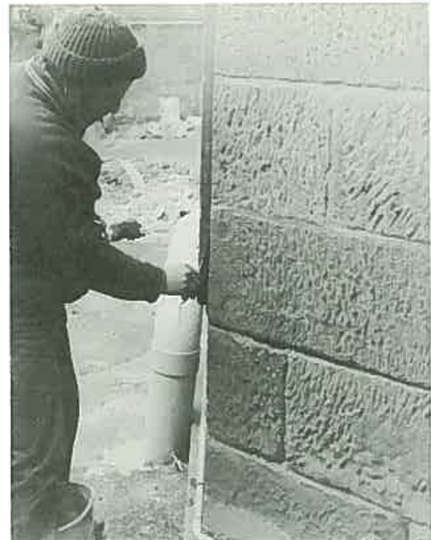
Mason raking out hard cement pointing prior to refacing certain stones and repointing the wall in lime mortar. (Government House, Hobart.)
