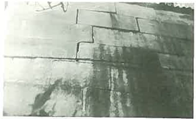
Structural movement such as this will probably mean the services of an engineer are required. (Goldfinders, Kurrajong, N.S.W.)
