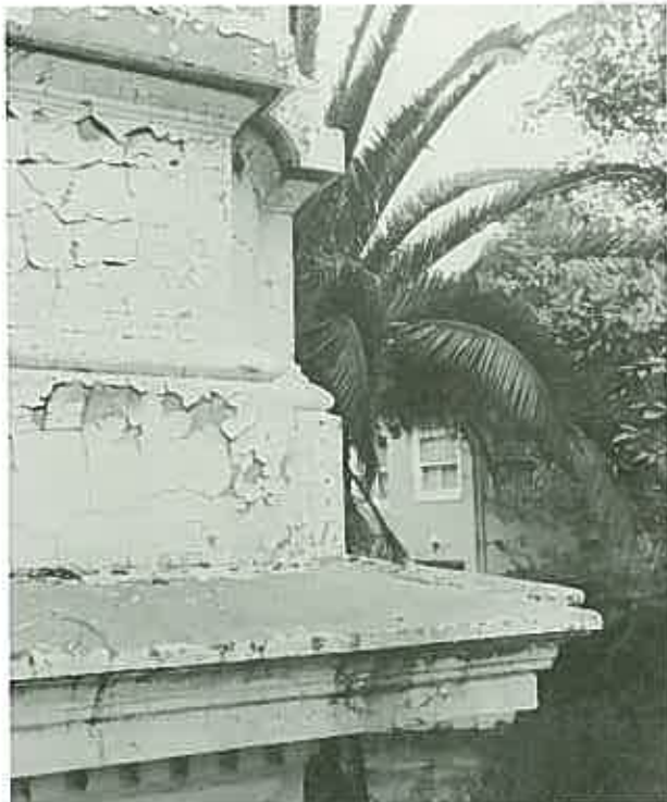
The masonry walls are cement rendered and marked out to look like detailed stonework. (Iona, Darlinghurst, Sydney, 1890.)
