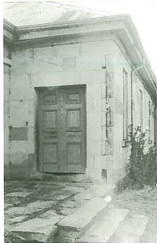
The original front doorstep to this house is very worn but if not sufficiently worn to have become dangerous or a problem, it should be kept. ( Bona Vista, Avoca, Tasmania. )
