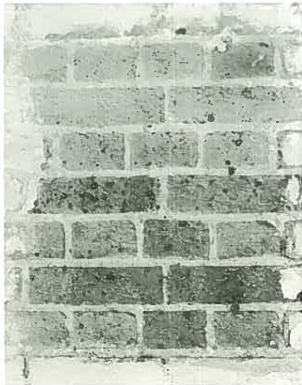
Cleaning paint off sandstock brickwork by a chemical and mechanical method removes the paint satisfactorily but the saturation of the wall may cause harmful chemical action with salts in the structure.
