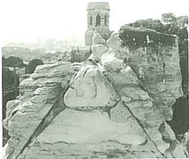
Exposed Sydney sandstone after a century of weathering in an urban environment. ( St. Andrew's, Balmain, 1855. )
