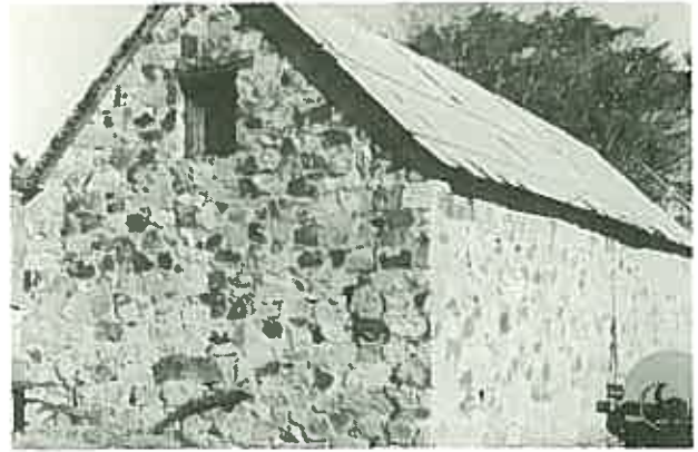
A good example of typical random rubble construction. The walls have once been limewashed so it should be understood the original quality was somewhat different. (Barn, Carcoar, N.S.W.)
