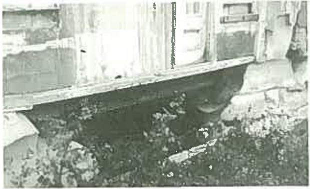
Advanced decay at a cellar opening caused by draught on severely salt contaminated masonry. (Lyndhurst, Sydney.)
