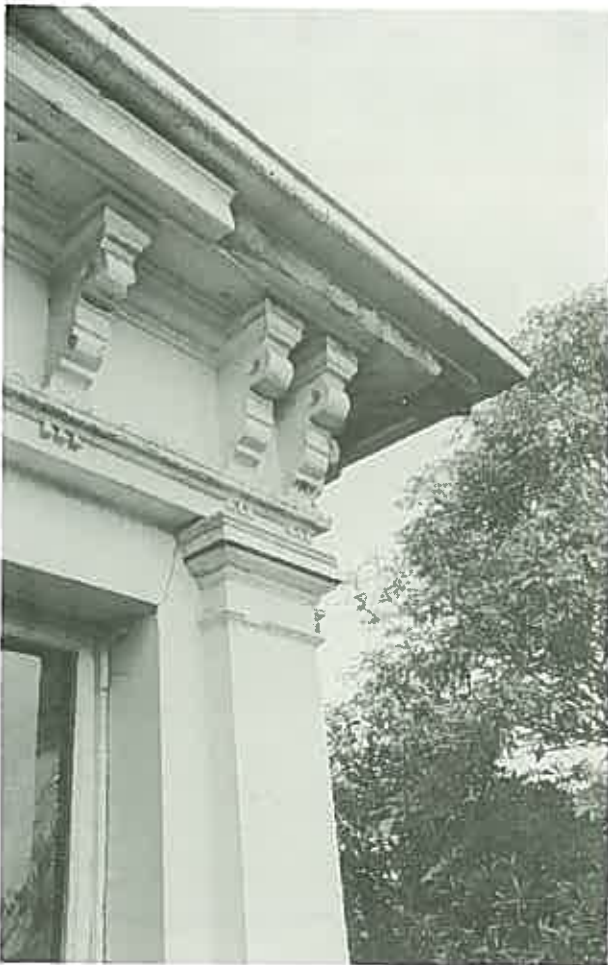
In this late Victorian house the cement rendered cornice has a core of sandstone. ( Iona, Darlinghurst, Sydney, 1890. )
