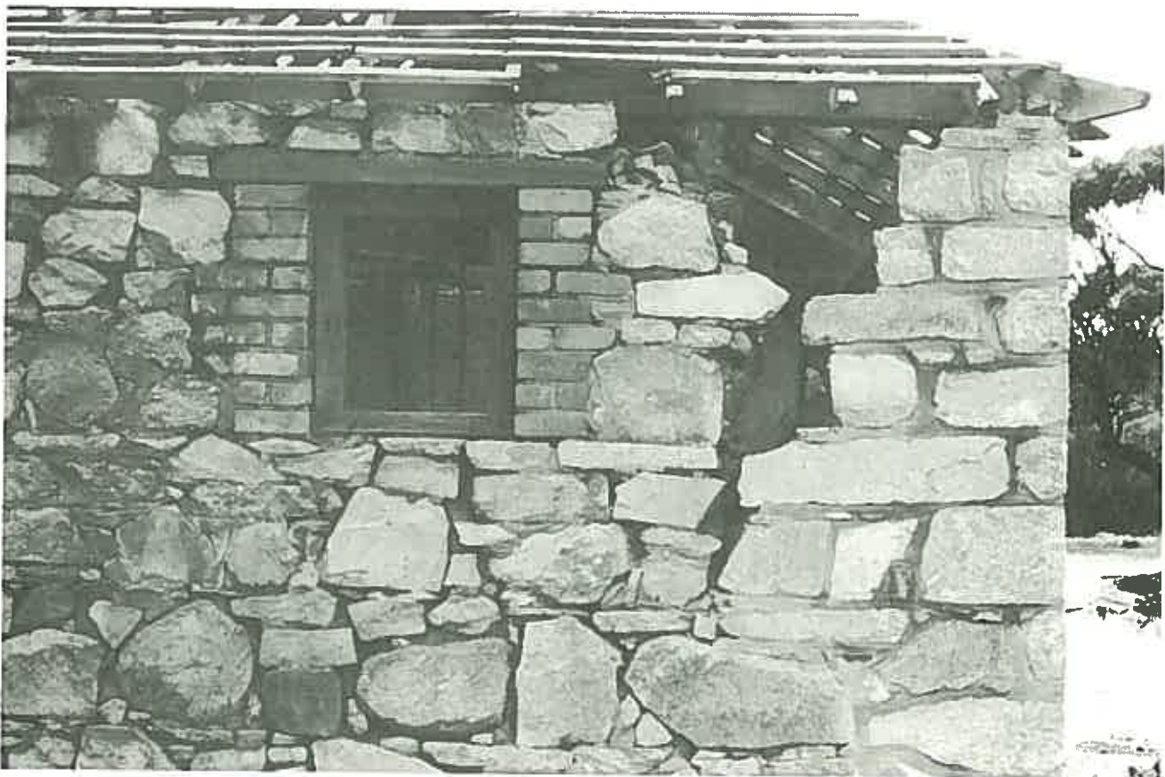
In this wall the repair has not captured the spirit of the original construction. ( Balladong, York, Western Australia. )
