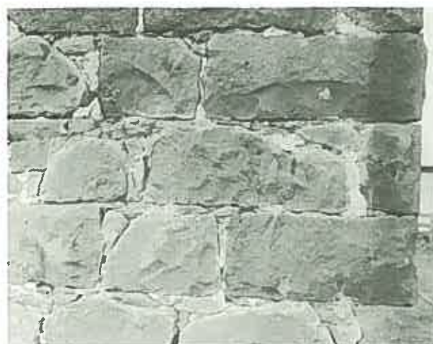
Fine bluestone rubble walling which has been squared and coursed in this western district example. (Shearing shed, Lyne Station, Hamilton, Victoria.)
