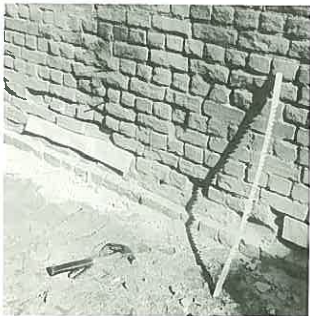
Cutting in a dampcourse in a 9" wall by the means of a masonry saw. (Cooma Cottage, Yass, N.S.W.)
