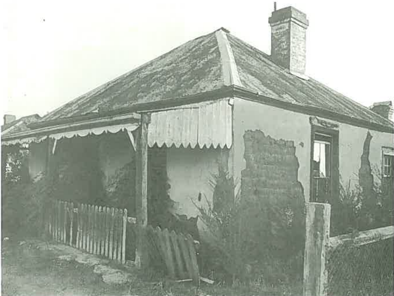
The rendering has broken down revealing that the cottage is of pise construction. ( Canowindra, N.S.W. Photo: Ian Stapleton. )
