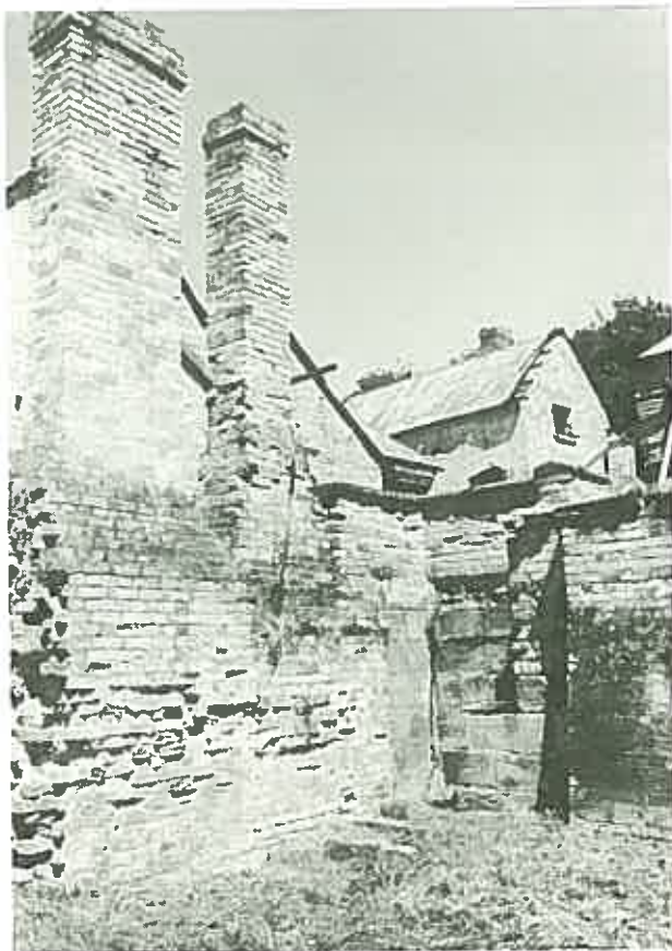
Severely neglected brickwork in which the effects of rising and falling damp can be seen. ( Commandant's House, Port Arthur. )
