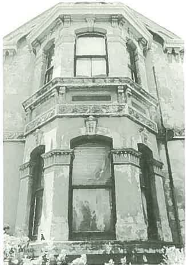
A late Victorian brick house encased in elaborate cement decoration. (House, 3 Arundel Street, Glebe, Sydney.)
