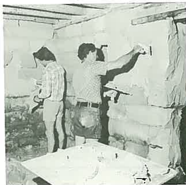
Fitting sacrificial plaster to salt contaminated walls will draw off the salt. (Cellar walls, Lyndhurst, Sydney.)
