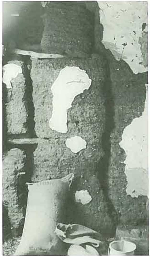
In this deteriorated pisé wall the timber reinforcing is seen. ( Stables, Boree Cabonne Homestead, Boreore, N.S.W. )
