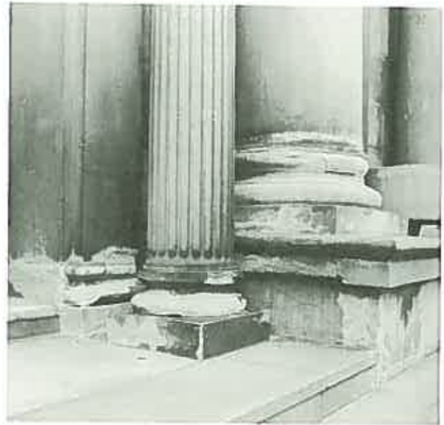
The effects of inappropriate repairs and rising damp. (Pitt Street, Parish Church, Sydney.)
