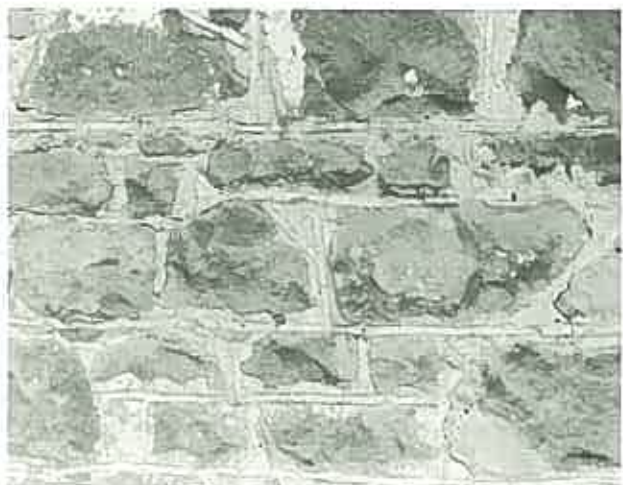
An example of rubble walling improved in appearance by the ironing of the mortar joints. ( Lyne Station, Hamilton, Victoria. )
