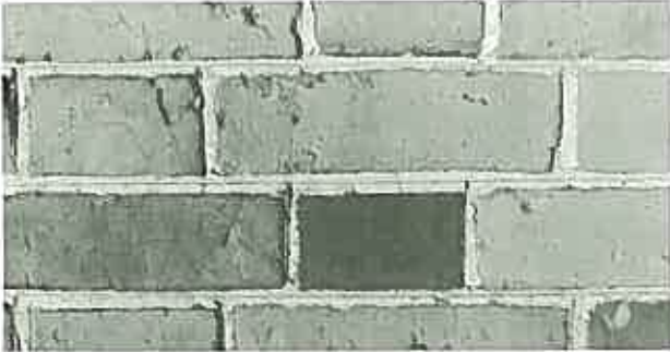
An example of pointing which has been ironed to make the joints appear finer than they are. This was a common 18th century practice. ( Forcett House, Fawcett, Tasmania, 1830s. )
