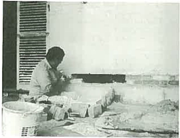
Cutting in dampcourse by removing sections of the wall. (Willandra, Ryde, Sydney.)
