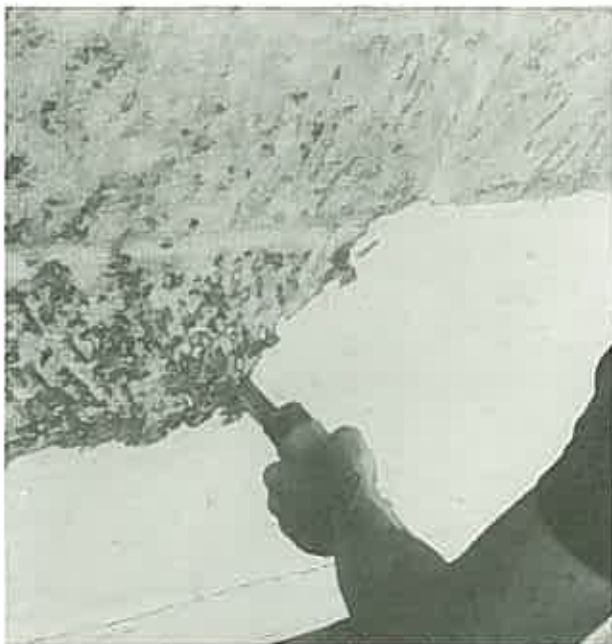
Removing paint off sandstone with a hand operated needle gun. It does not remove all the paint but in a few years what remains could well weather off.
