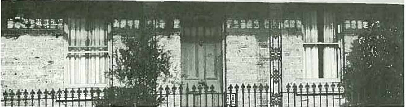
In recent years many 19th century buildings have had their protective render coat removed to expose the sandstock brickwork in the mistaken view that this is how they were originally. (45 Moncur Street, Woollahra, Sydney. Photo in possession of Mrs. S. Carter.)
