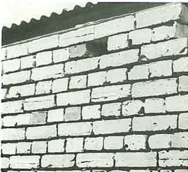
This shows the beneficial effects of a soft mortar. In this neglected wall the mortar has gone and left the bricks intact. ( Outbuilding, Parsonage, Port Arthur, Tasmania. )
