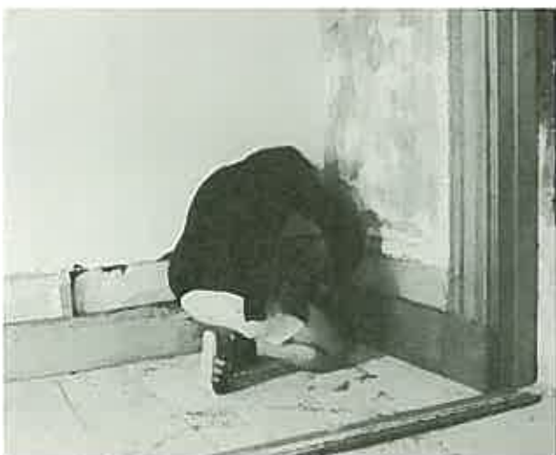
Architraves and skirtings are fitted to protect the soft plaster. ( Lyndhurst, Sydney. Restoration architect: Clive Lucas. )
