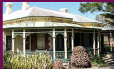
ABOVE: The deteriorated verandah roof at Samson House is expected to be replaced by the end of June. M Dossin
