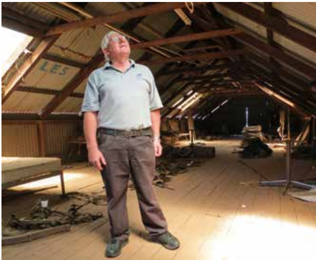
ABOVE: Conservation Project Officer Eric Hancock inspects the roof space of the old Avondale stables. R Bishop
