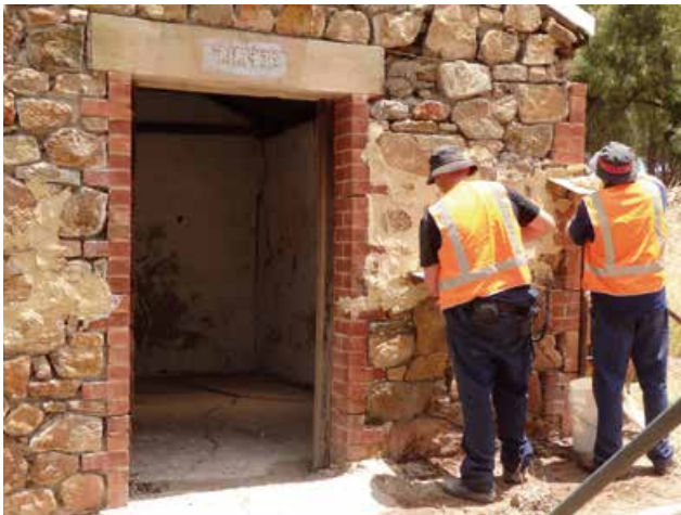
ABOVE: The program provides training in lime mortar skills and delivers immediate conservation outcomes. S Murphy
