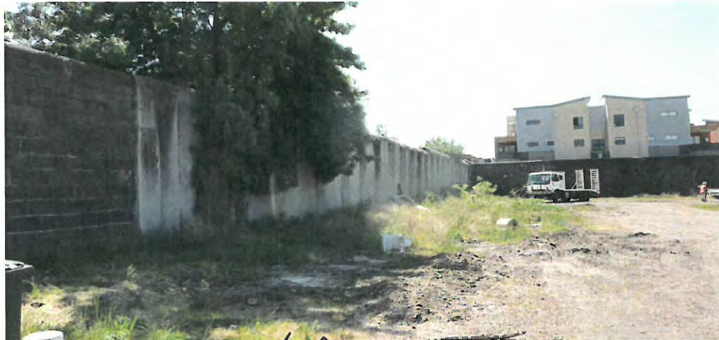
Figure 13 The subject site: view of the west wall, part of which is enclosed in reinforced concrete
