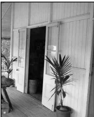
Style of exposed framing showing belt rails and internal VJ boards, introduced
