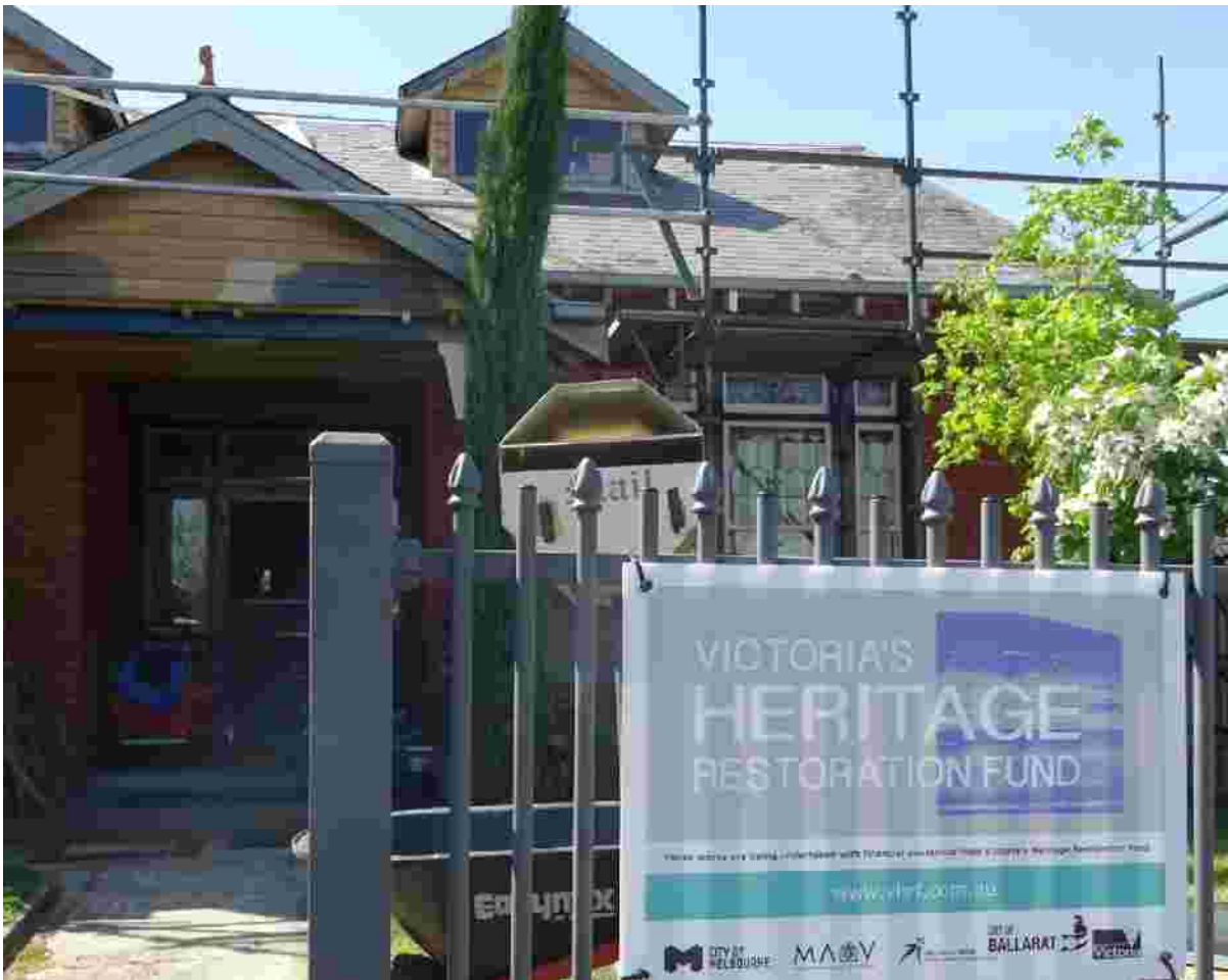
Replacement of a slate roof funded through the Victoria's Heritage Restoration Fund .
