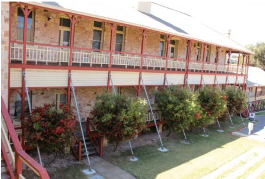
ABOVE: Works are scheduled for the veranda at Crowley House in early 2014. E Hancock NTWA
