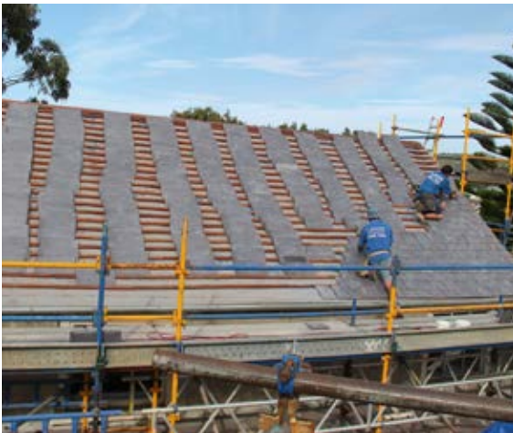
ABOVE: New time lapse movie captures the reroofing process in spectacular fashion at Old Farm, Strawberry Hill. E Hancock NTWA
