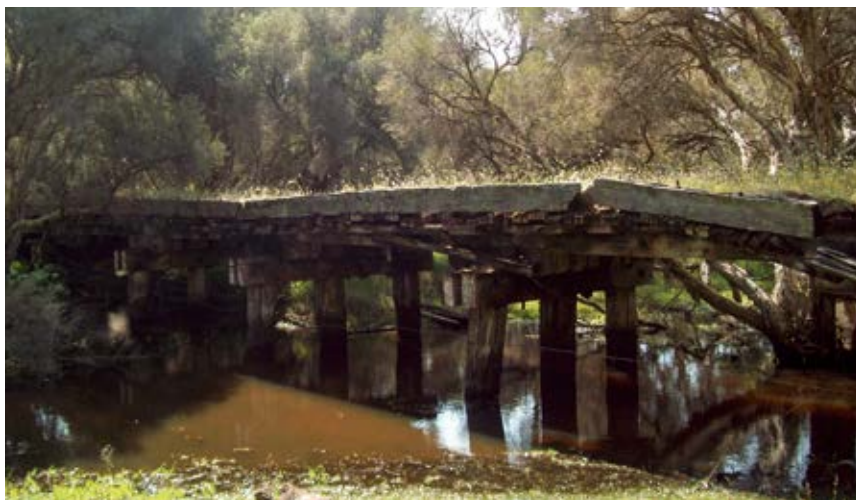
ABOVE: Kangaroo Gully Bridge is one of only four bridges which is salvageable along the trail. Water Corporation. The bridge will support pipework and well as pedestrian and cyclist traffic when restoration work is complete. Water Corporation
