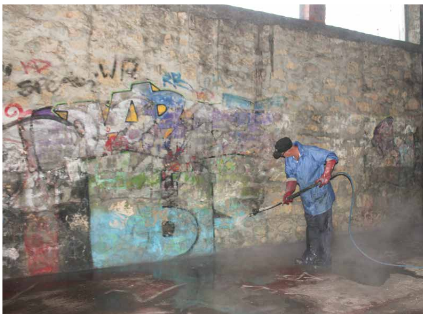
ABOVE: Phillip King from Abel Wasserman tackles the substantial graffiti damage at Luisini Winery. M Dossin
