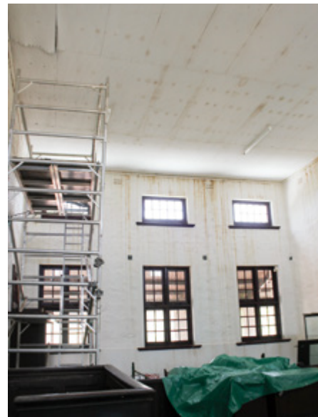
ABOVE: View showing mobile scaffolding to inspect the roof inside the former Courtroom, a George Temple Poole designed building, 1885/1886. C Stokes
