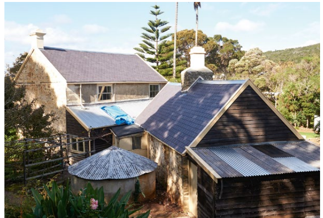
ABOVE: One of the 30,000 frames shot as part of an innovative time-lapse production which has captured the roof conservation process. G Pickering NTWA
