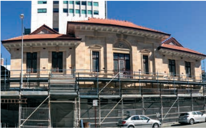
ABOVE: The conserved facade of 57 Murray Street is revealed as the scaffolding comes down. Western Projects
