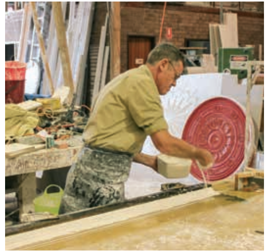
ABOVE: David Wallace from Chris Savage Plaster Design runs a new cornice to conserve and restore the original cornices at 57 Murray Street. C Stokes NTWA
