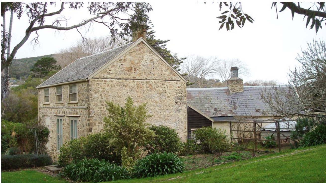
ABOVE: The National Trust is undertaking research to inform the replacement of the slate roof at Old Farm, Strawberry Hill. NTWA
