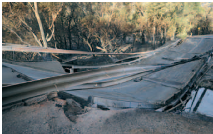
Buckingham Bridge was severely impacted by recent fires. L Margetts
