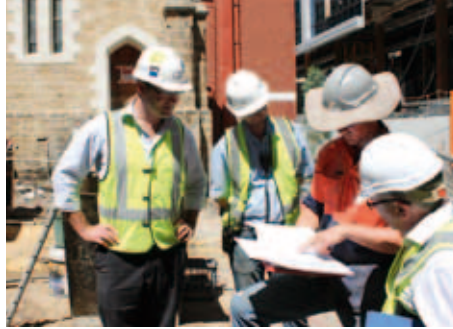
Engineers confer at the Old Perth Boys' School in St Georges Toe, Perth. National Trust/E Hancock
